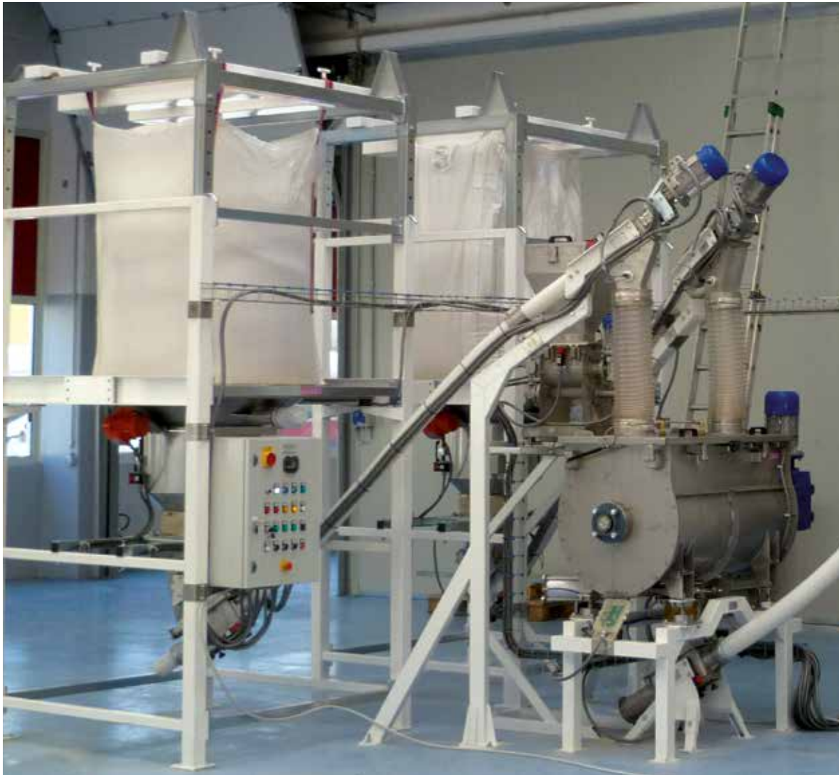
Bulk Bag Unloading with Flexible Screw Conveyors, Dosing, Batch Mixing of three different components and Conveying into buffer silo
